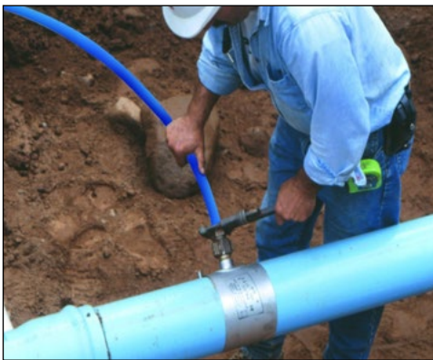
Figure 10.13 PEX Tubing Installed with 10- to 20-Degree Gooseneck
